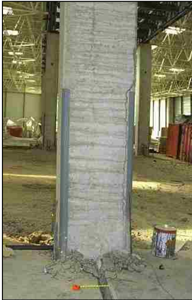
Figure 3.35 Longitudinal cracking: earthquake damage (PEER)
