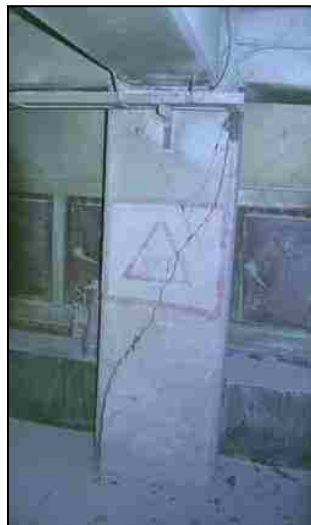
Figure 3.73 Widening and localization of shear cracks: earthquake damage (PEER)
