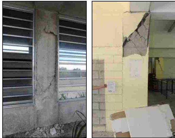
Figures 3.71 and 3.72 Widening and localization of shear cracks: earthquake damage (Eberhard, et al. 2010)
