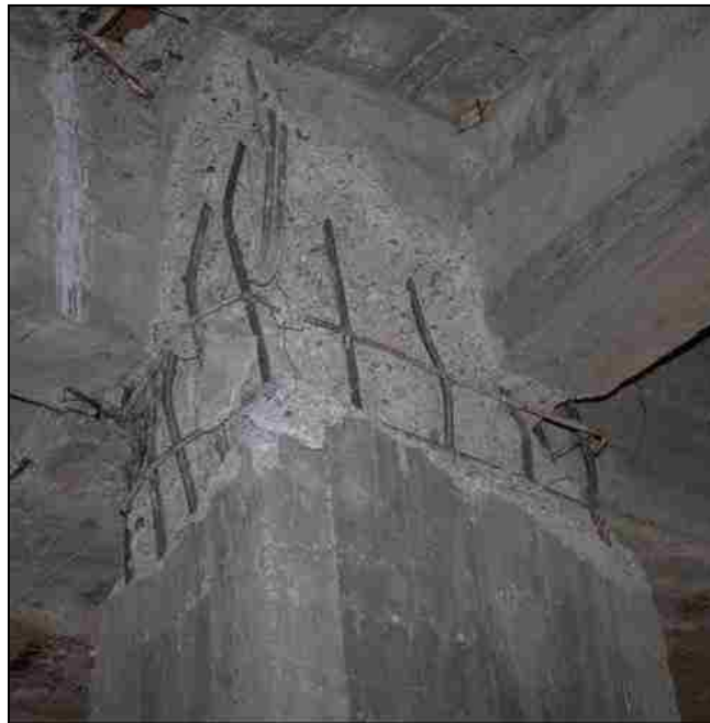
Figure 3.54 Crushing of core concrete: earthquake damage (PEER)
