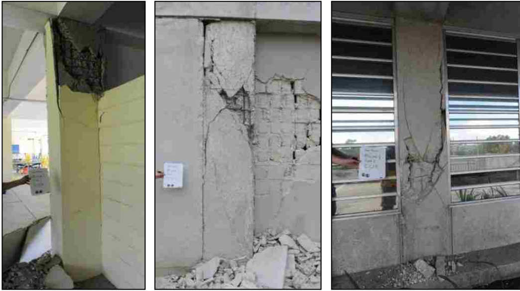
Figures 3.84, 3.85, and 3.86 Concrete spalling on side faces: earthquake damage (Eberhard, et al. 2010)
