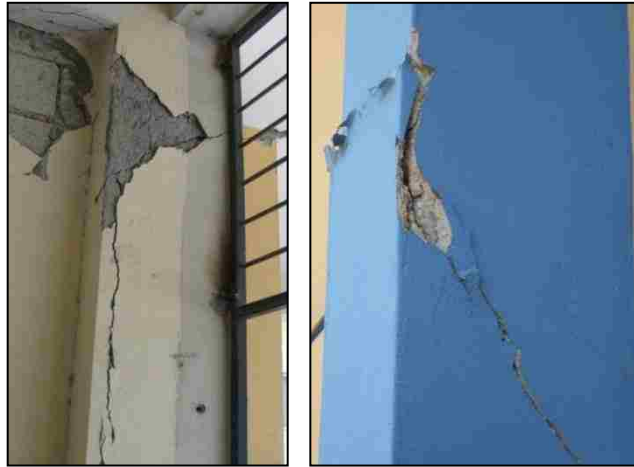
Figures 3.69 and 3.70 Widening and localization of shear cracks: earthquake damage (Sedra, et al. 2010)
