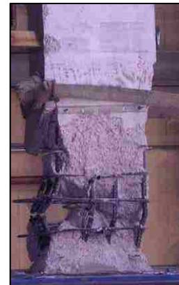
Figure 3.21 (F8) Longitudinal Bar Fracture
