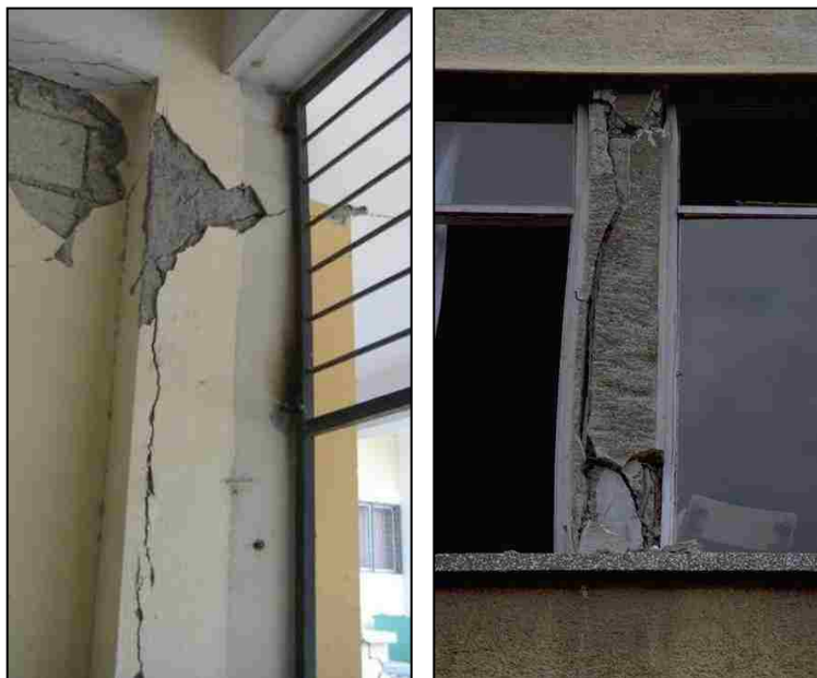
Figures 3.76 (Sedra, et al. 2010) and 3.77 (PEER) Longitudinal cracking on side faces: earthquake damage
