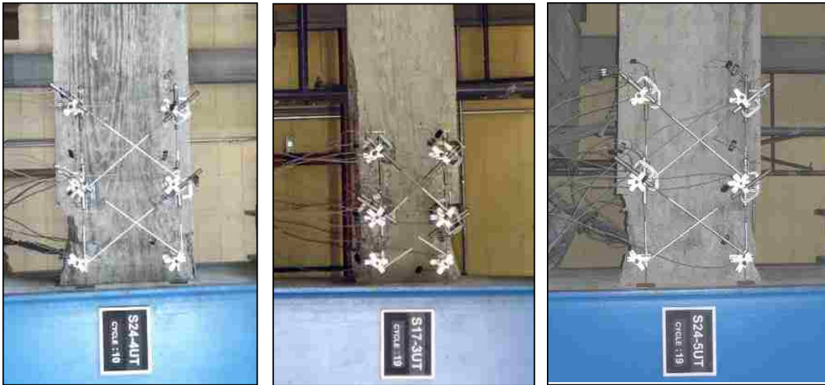
Figures 3.37, 3.38, and 3.39 Concrete spalling on flexural and side face: experimental damage (Bae 2005)
