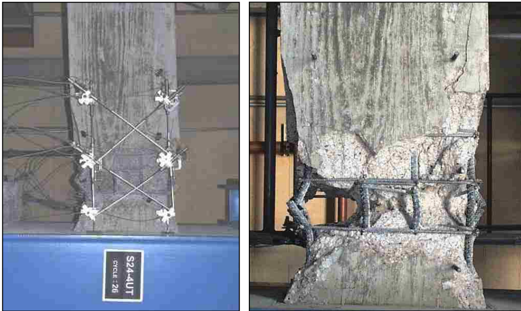
Figures 3.55 and 3.56 Longitudinal bar fracture: experimental damage (Bae 2005)
