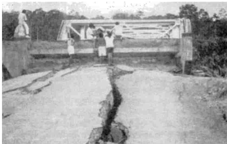
Figure 1.3: Settlement and longitudinal cracking of southern approach embankment at Rio Estrella Highway Bridge (Youd, 1993).
