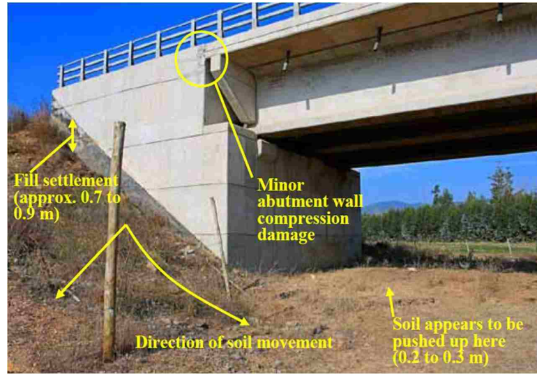
Figure 1.4: Settlement and lateral spreading deformation of northeast approach embankment to Mataquito River Bridge (FHWA, 2011).
