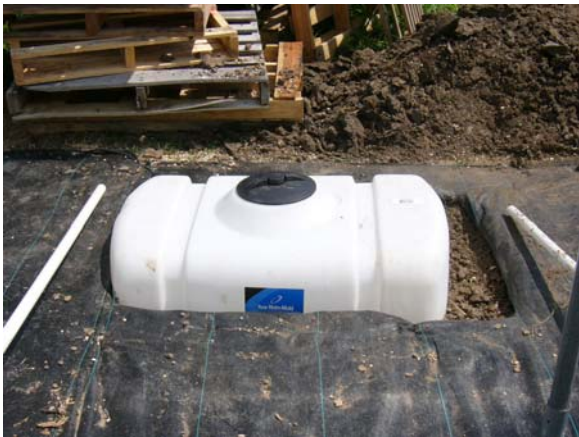
Figure A-9. Discharge Sump Tank
