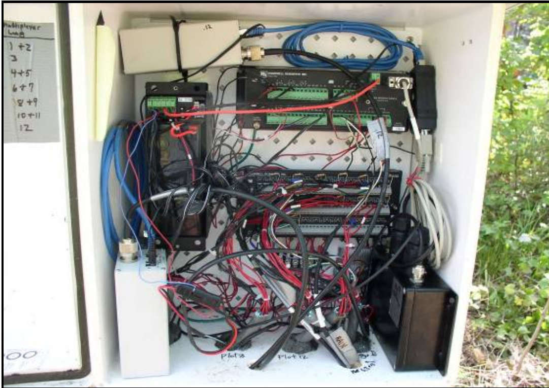
Figure 3.6. Primary site data logging station with Campbell Scientific CR-10X ® datalogger, CSI AM16/32 multiplexer, radio telemetry, satellite uplink, and atmospheric environmental monitoring equipment.
