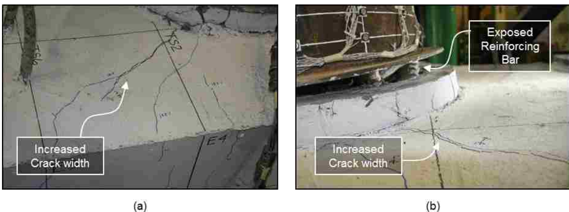
Figure 5.45: WRCUB South (a) cap beam cracking, and (b) exposed reinforcing bar at 8.19% drift North
