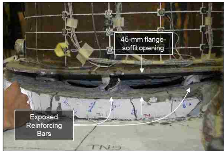
Figure 5.46: WRCUB North exposed reinforcing bars at 9.76% drift South
