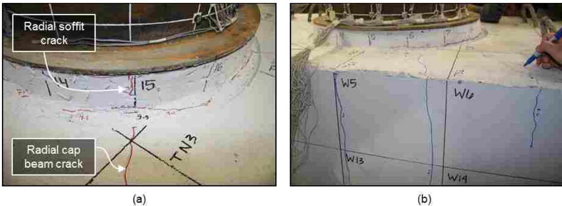
Figure 5.18: WRC radial cracking on (a) North side of column at 1.48% drift, and (b) south side of column at 1.62% drift
