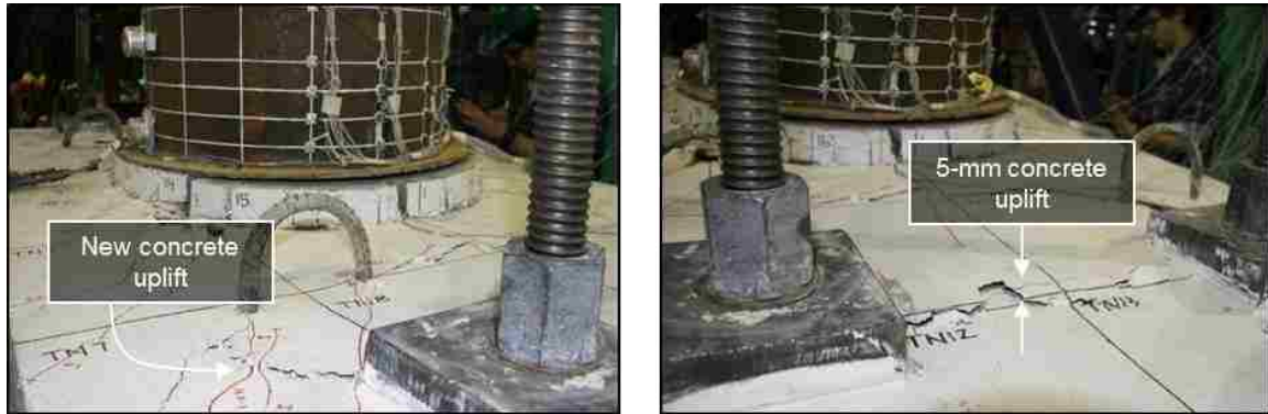
Figure 5.32: WRC North cap beam uplift at 9.71% drift South (Cycle 2)
