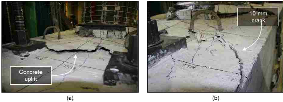
Figure 5.35: WRC South cap beam (a) uplift and (b) cracking at 11.01% drift North
