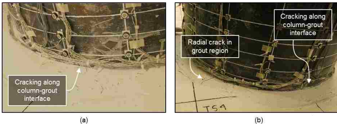
Figure 5.64: EMB96 (a) North and (b) South grout pad cracking at 0.5% drift
