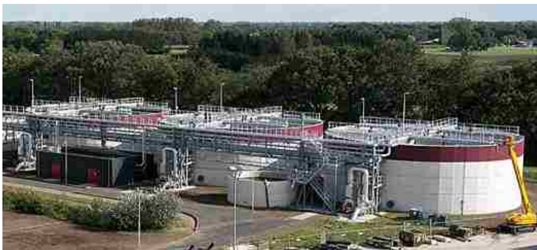
Figure 7-3. Aerial image of Nereda® Plant in Epe, The Netherlands. Reprinted with permission from the Netherlands Water Partnership. Copyright Netherlands Water Partnership. Retrieved from http://www.dutchwatersector.com/news-events/news/2704-official-commissioning-nereda-at-wwtp-epe-wonder-granule-keeps-its-promise.html
