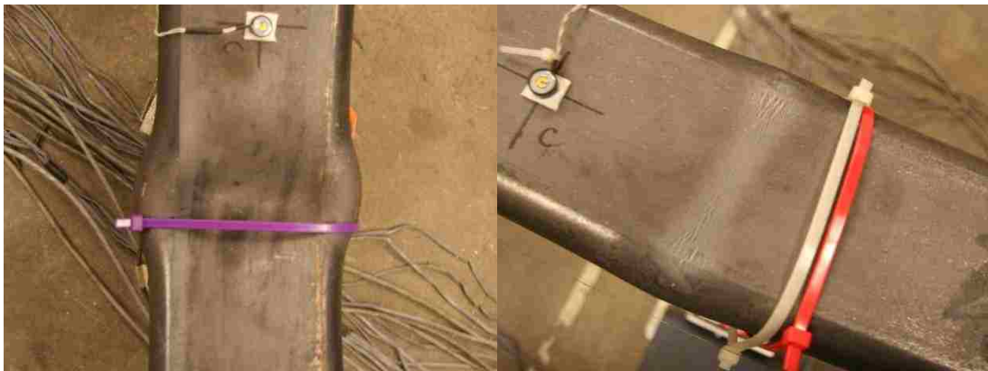
Figure 4.23: Severe local cupping of N brace (left) and initial tearing of S brace (right) at +3.0% drift.
