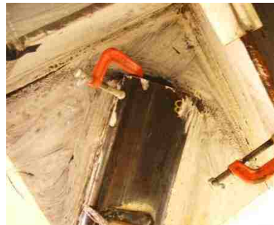
Figure 4.36: Mid-span GP yielding at -0.83% drift.
