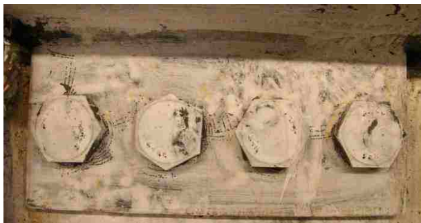
Figure 4.35: Shear tab yielding at 0.83% drift (Y1).
