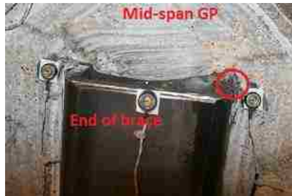
Figure 4.12: GP crack at N brace-to-gusset weld (PC1).
