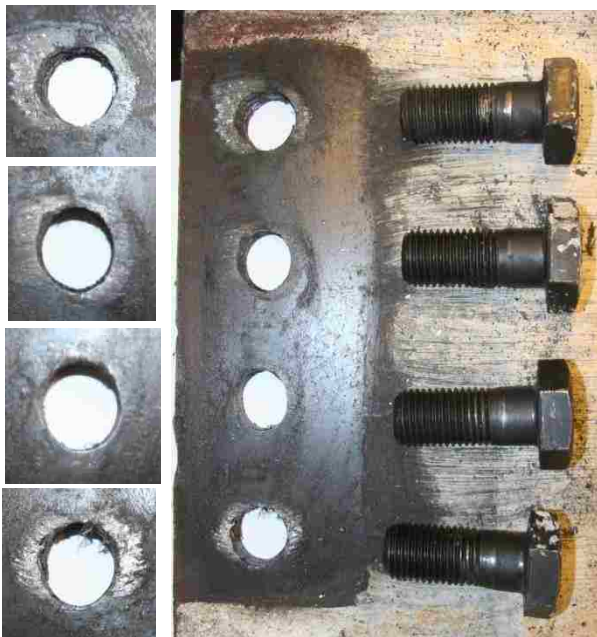
Figure 4.90: S beam web bolt hole elongation.
