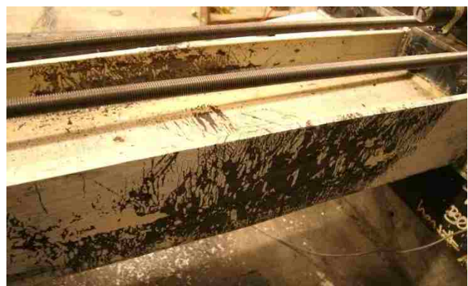
Figure 4.49: S col. severe yielding at 2.8% drift (Y3-OF/IF).
