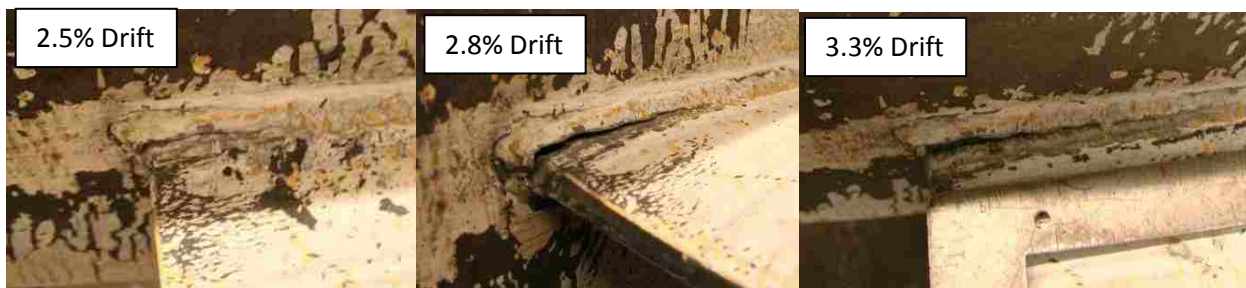
Figure 4.19: Crack propagation in NE corner gusset-to-column weld (WT1,2,3).
