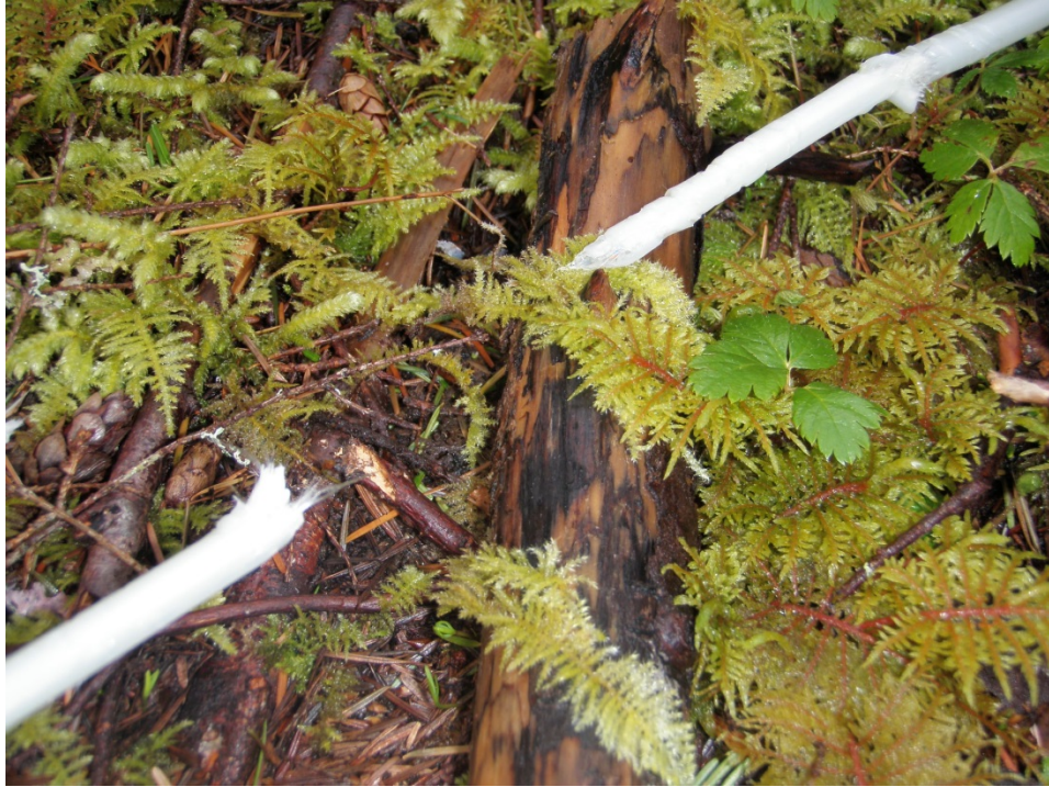
Figure 3.10 Photograph of bear damage to the fiber-optic cable.
