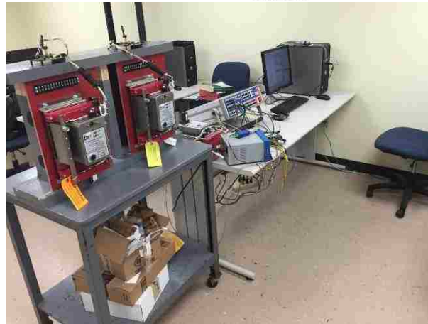
Figure 4.2: LV secondary network grid vault connected to two feeders and a lab test setup
