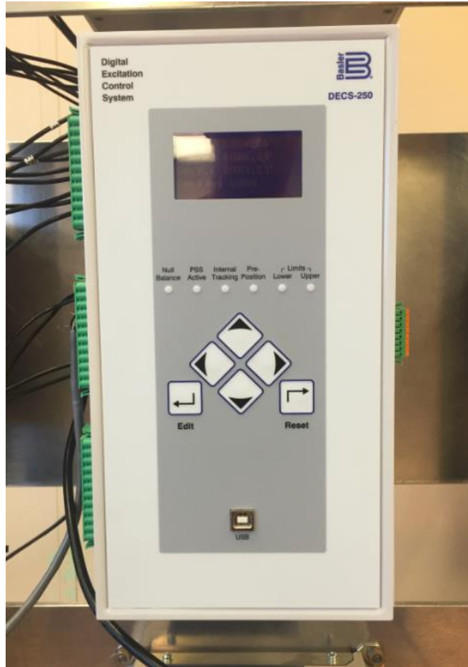
Figure 3.4: Generator Voltage Regulator
