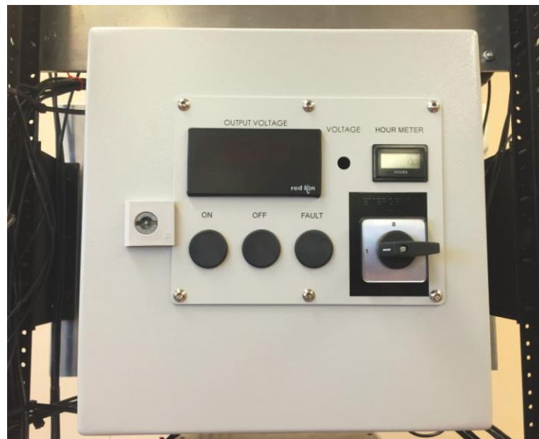
Figure 3.2: Generator Impedance Switch
