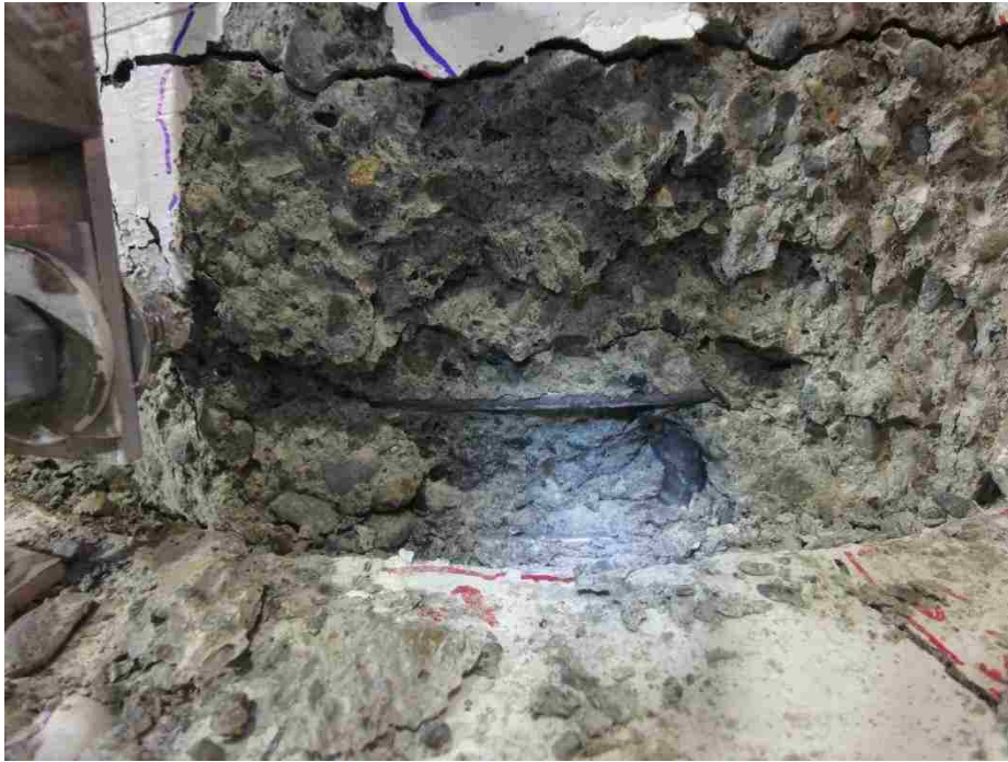
Figure C-0-17. DS-3 – First noticeable bar buckling in the column at 5.59/-7.00 percent drift
