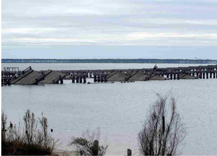
Figure 1-6: The Biloxi Bay Bridge after Hurricane Katrina (Douglass et al. 2006)
