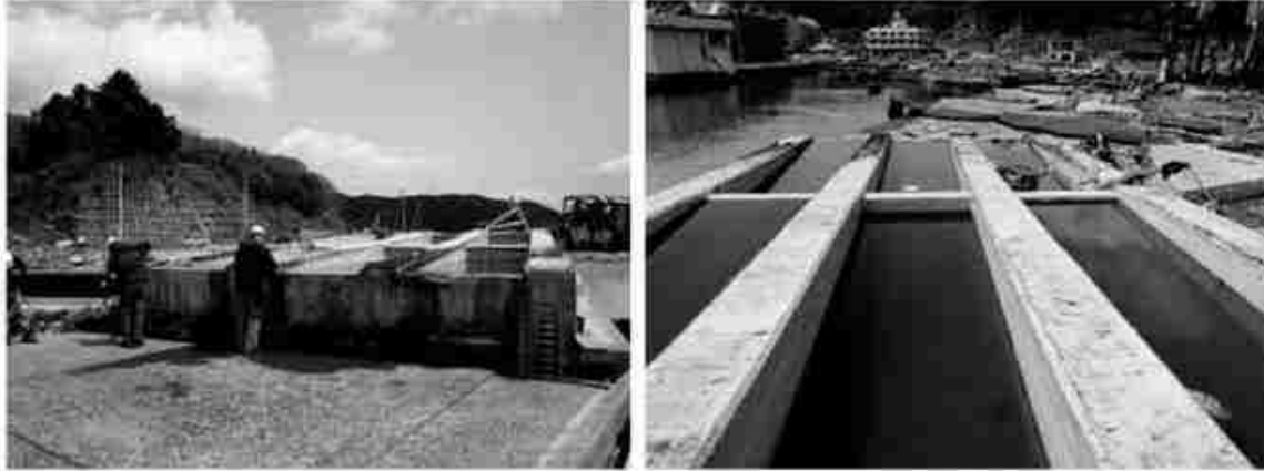
Figure 1-5: Flipped Bridge Superstructures due to the 2011 Great East Japanese Earthquake and Tōhoku Tsunami (Chock (left) & Robertson (right), with permission from ASCE)
