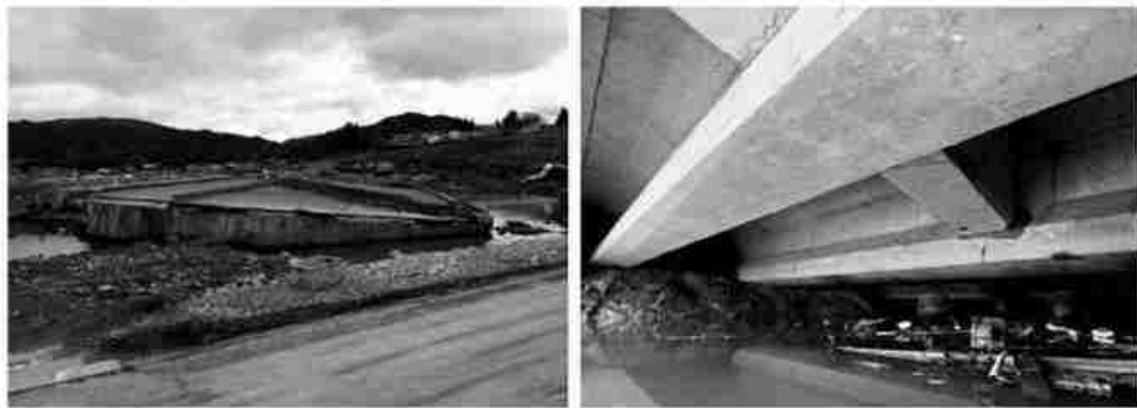
Figure 1-3: Deck Section Displaced from Original Location due to the Uplift (2011 Great East Japanese Earthquake and Tōhoku Tsunami, Robertson, with permission from ASCE)
