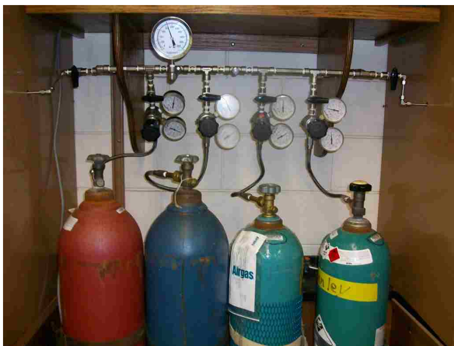
Figure 2.10. Current gas manifold design.
