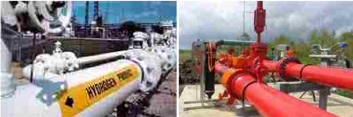
(a) Hydrogen pipeline in USA
