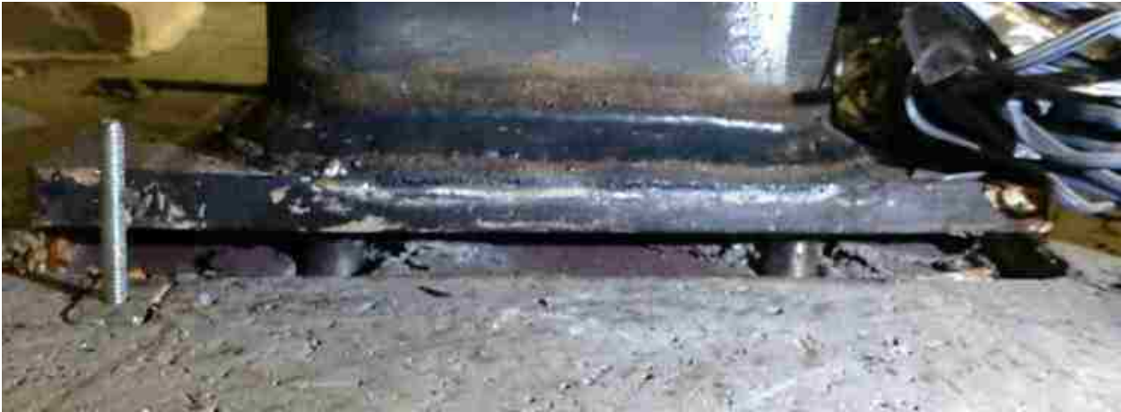
Figure 6.5.5.4: Concrete profile around the studs after failure (Specimen 2-2-0.50)
