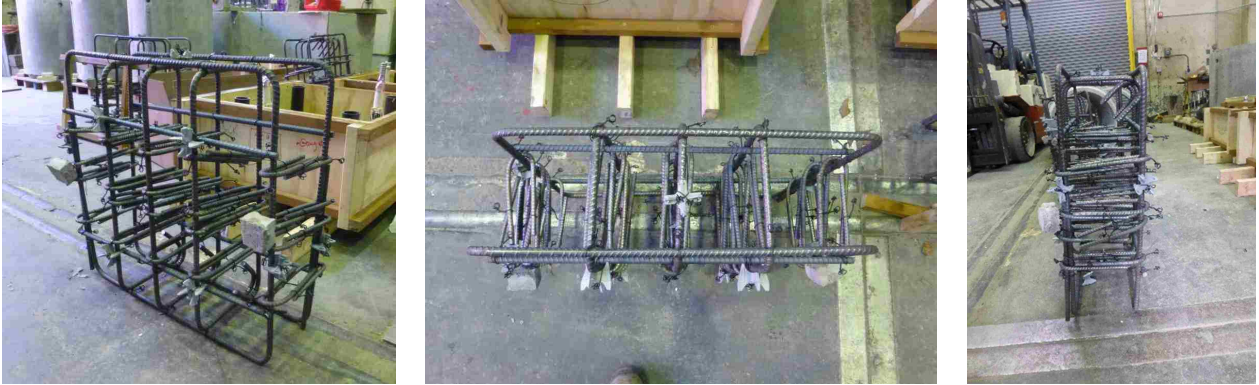
Figure 6.2.1.4: Reinforcement cage side by side views
