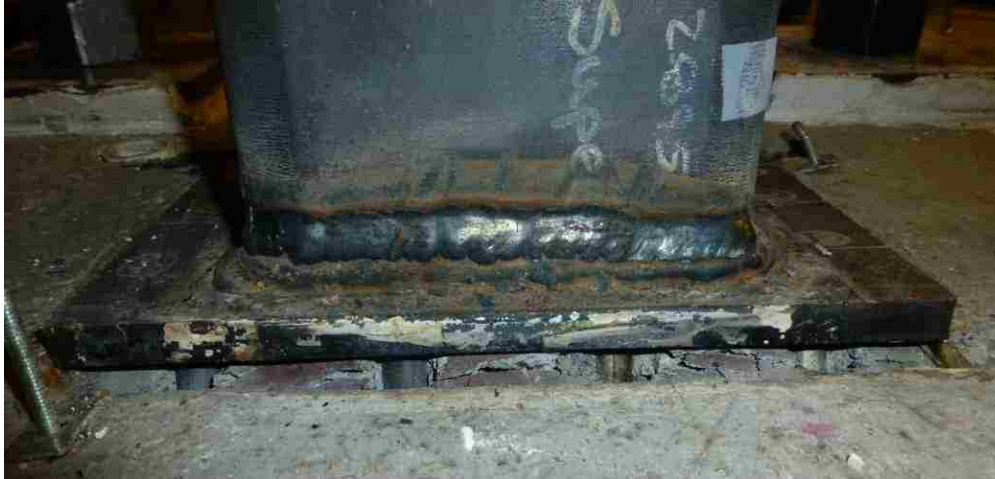
Figure 6.5.2.5: Concrete profile around the studs after failure (Specimen 4-0-0.92)
