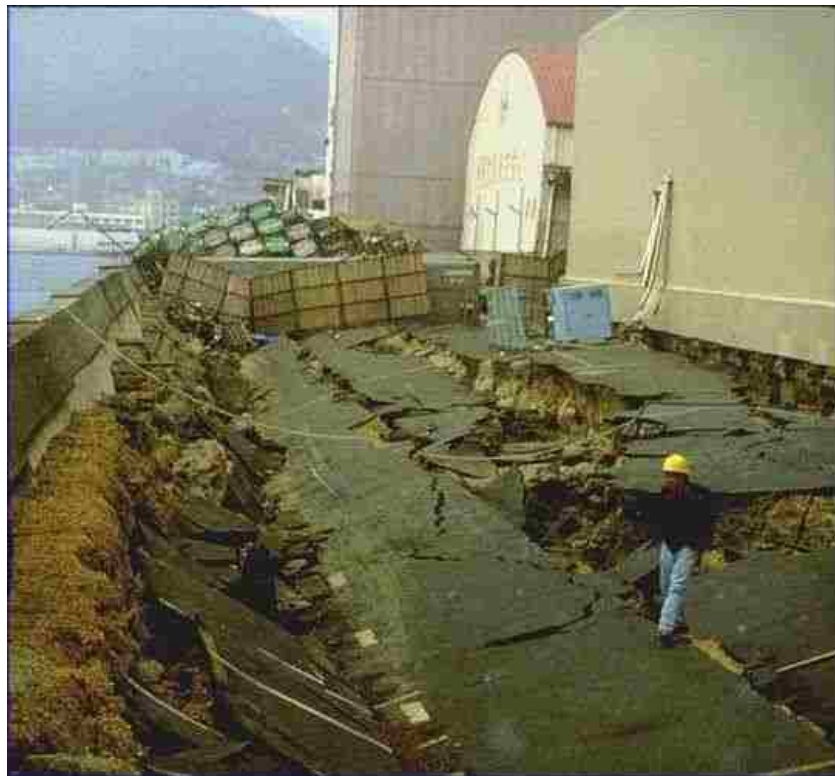
Figure 5.2. Liquefaction-induced lateral spreading from the 1995 Kobe, Japan earthquake causing severe damage to a quay wall (UW).
