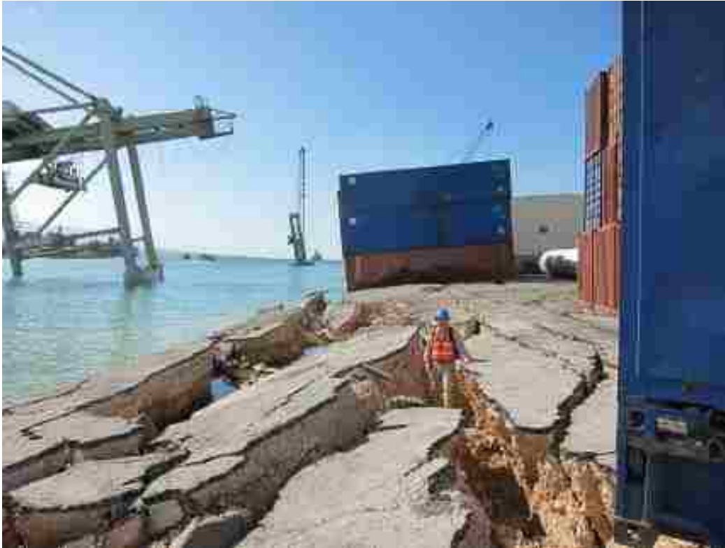
Figure 2.2. Liquefaction-induced lateral spreading at the North Wharf of the Port de Port-au-Prince (photo from DesRoches et al., 2011).
