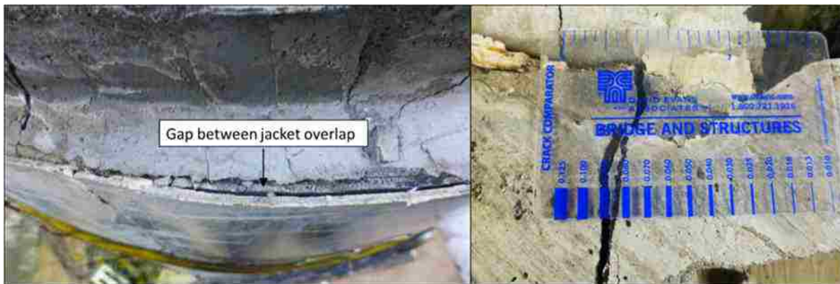
Figure 5-18. Observations at the end of Test 12-ep24s1-1 including gap opening and crack width at the top of the specimen
