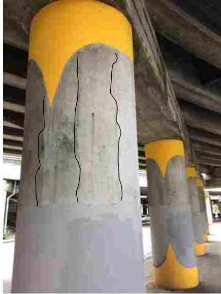
Figure 1-2. Longitudinal cracks on columns of Ravenna Bridge
