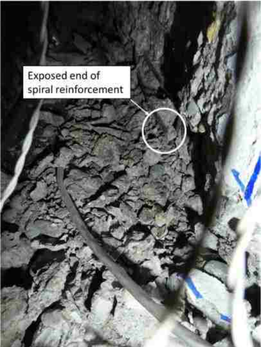
Figure 8-9. Substantial spalling at base of column, Series 7
