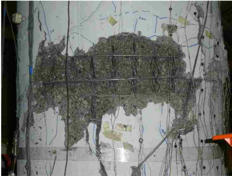
Figure 9-3. "Damaged Area" at end of testing showing concrete spalling, buckled strands and spiral deformation
