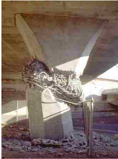
Figure 2.4: The flared piers of the Mission-Gothic underpass experienced shear failure during the 1994 Northridge Earthquake, likely after yielding of the longitudinal reinforcement reduced the pier's shear capacity [5].
