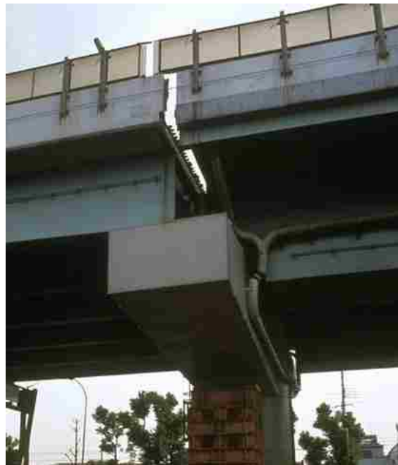
Figure 2.3: Differential movement between adjacent deck sections at an expansion joint led to a span discontinuity at pier 97 of the Hanshin Expressway in Japan after the 1995 Kobe Earthquake [55].
