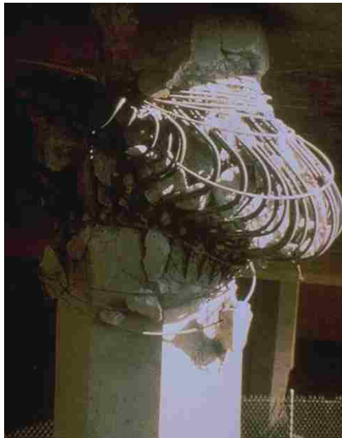
Figure 2.5: Inadequate confinement in the I-10 La Cienega-Venice overpass led to buckling of longitudinal reinforcement and crushing to core concrete during the 1994 Northridge earthquake [18].
