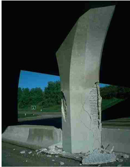
Figure 2.6: Unconfined concrete on the Ruffner Ave bridge spalled off during the 1994 Northridge earthquake [31].
