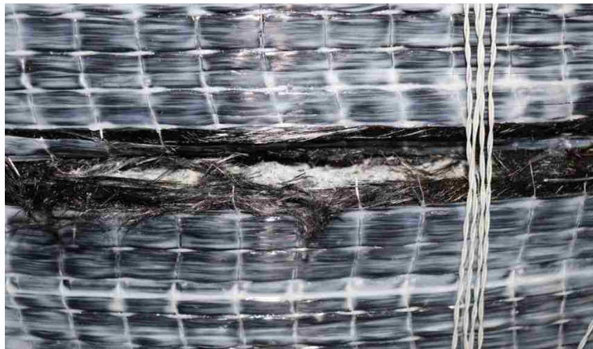
Figure 7-11. Close up view of split at 35-inches above cap beam
