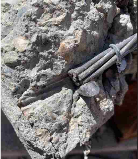
Figure 7-21. Strand slip at the base of the pile-column wall
