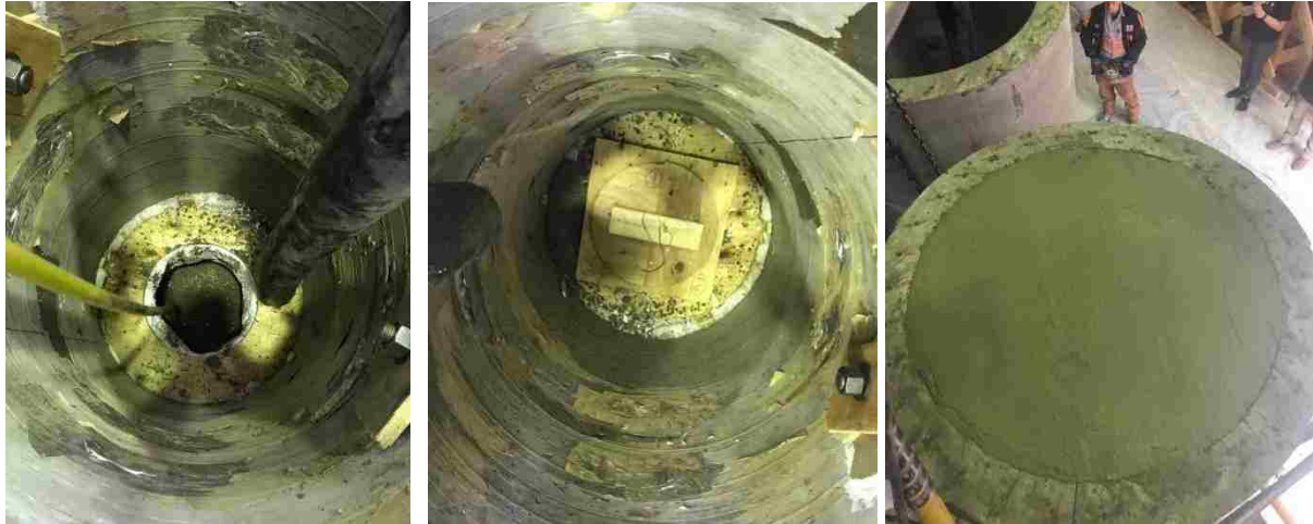
Figure 3-17. Left: Bottom half of fill concrete; Middle: Wood plug inserted; Right: Top half of fill concrete
