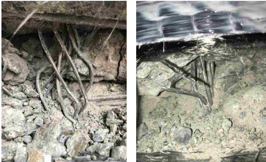
Figure 7-16. Buckled strand (left) and fractured strand (right)
