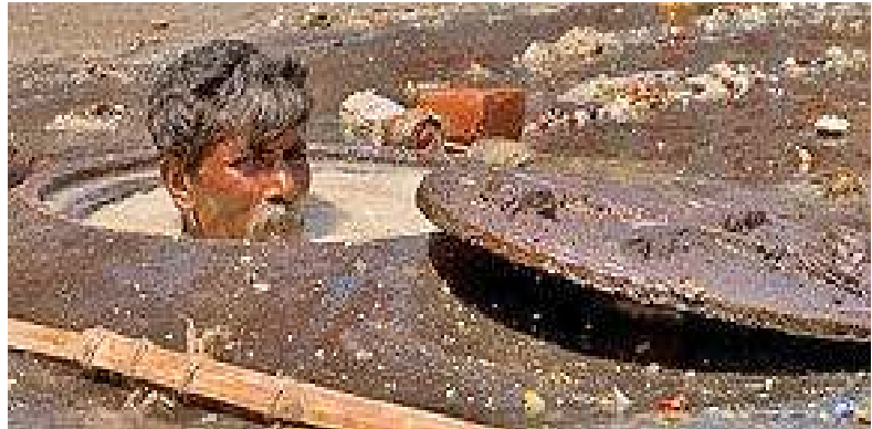
Figure 5. Man unclogging sewer overflow, Chennai, India
