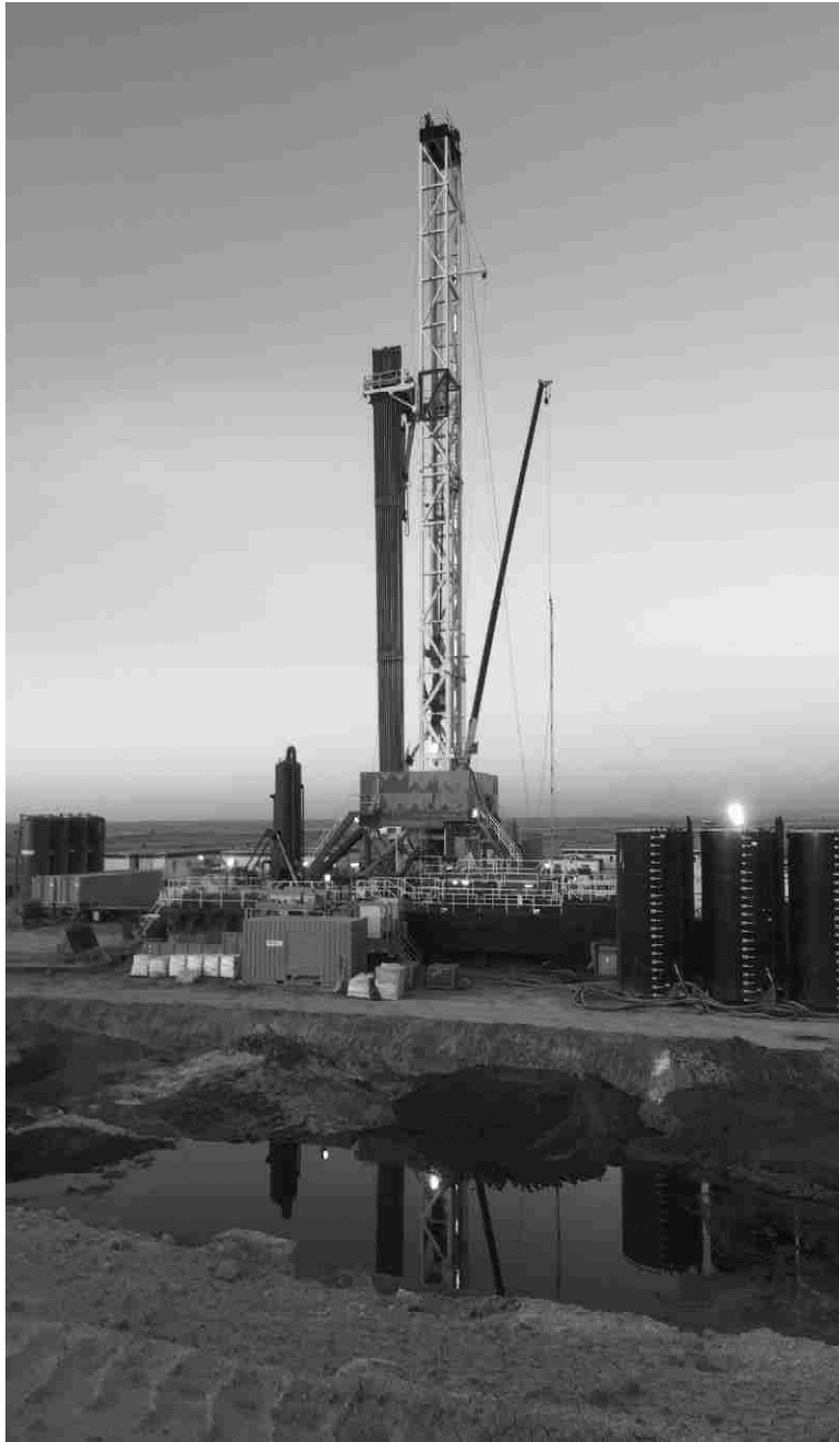
Figure 1: Sublette County, Wyoming: View of rig with cuttings pit in foreground. Notice the crane to the right of derrick: a second crew is on-site to perform fracking operations on a well that has already been drilled. They use the crane to lift the coiled-tubing that can perform the perforation of casing and send the frack-fluid downhole. This is known in the industry as Simops (Simultaneous Operations), the simultaneous drilling of wells, while also fracking wells on the same well-pad. In this case a four-well pad. Author's photo.
