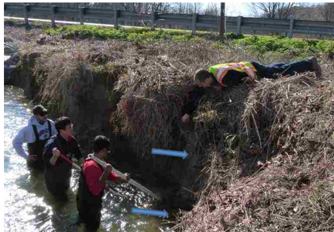
Figure 42. Installation locations of the lateral riverbed migration posts
