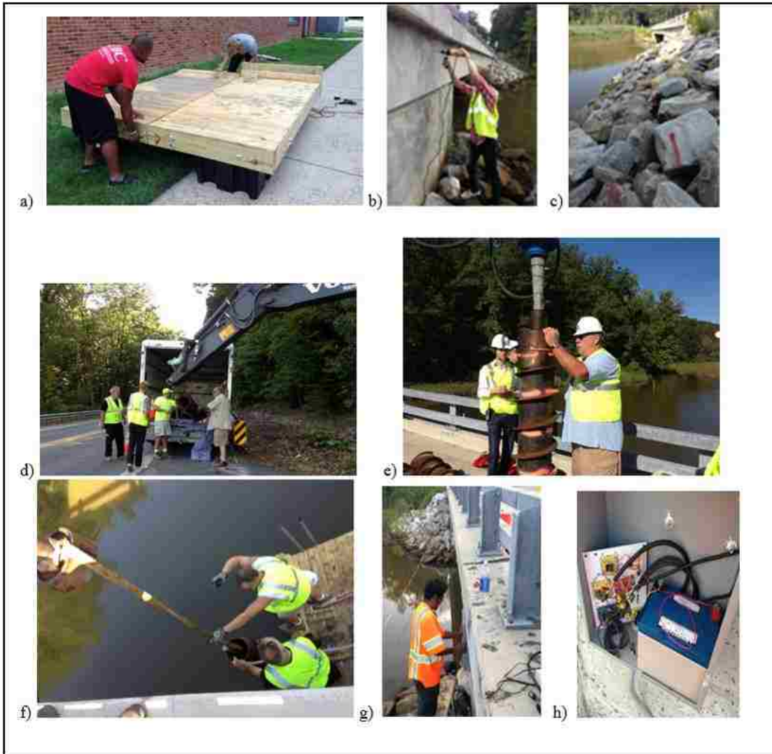
Figure 35. Photos of full-scale installation at Bridge No. 02072 on MD450 over Bacon Ridge Branch. a) students building installation working platform; b) installation of electronics housing on bridge structure; c) contact Miss Utility well in advance
