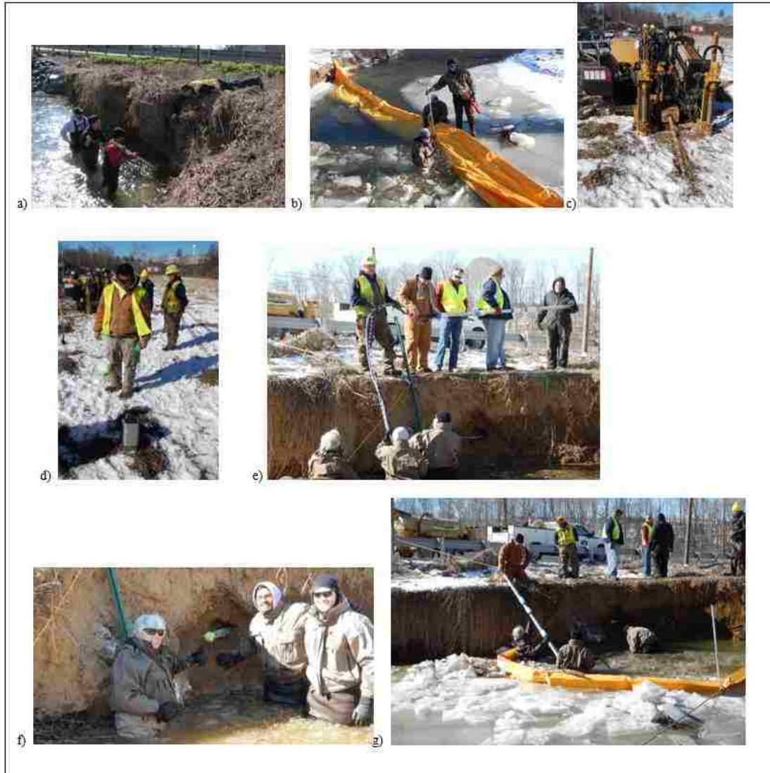
Figure 46. Photos of full-scale installation at Bridge No. 1008600 on MD355 over Bennett Creek. a) Jeff Knaub of MDSHA showing UMD students target location for sensors; Rip rap protecting bank from prior scour event at top left of photo; b) installation of turbidity curtain on morning of installation; c) BelAir drill rig ~9.2m (30 ft) from where sensor will protrude from bank; d) sensor used to track depth and lateral position of drill tip; e) feeding wiring and sensor post into bank ~60 cm (2 ft) above nominal water level as drill bit is retracted; f) admiring successful installation of the in-air sensor post; g) feeding wiring and sensor post into bank at depth of ~15.25cm (6 inches) below nominal water level for this site.
