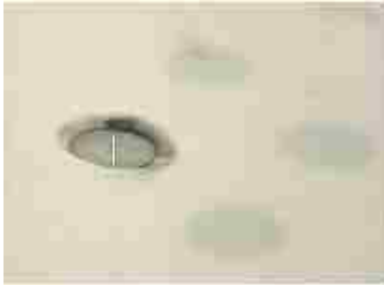
Figure 3.10: Close up of broken MACOR ® surface over a heat flux gauge showing the exposed thermocouple bead and leads. In the initial experiment configuration, this was repaired by covering with Bondo, a body filler to minimize disturbances to the flow.
