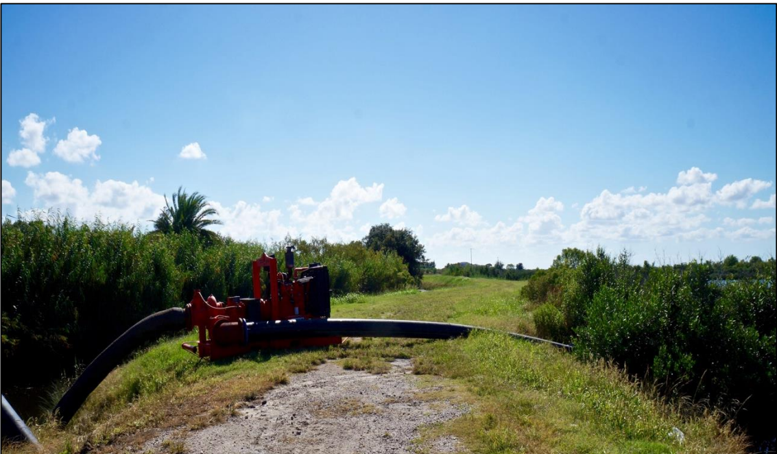
Image 10: A second pump on the tidal surge protection levee pumps floodwaters from the canal over the levee and back into the bay. Source: Miller, Lauren 2018.
