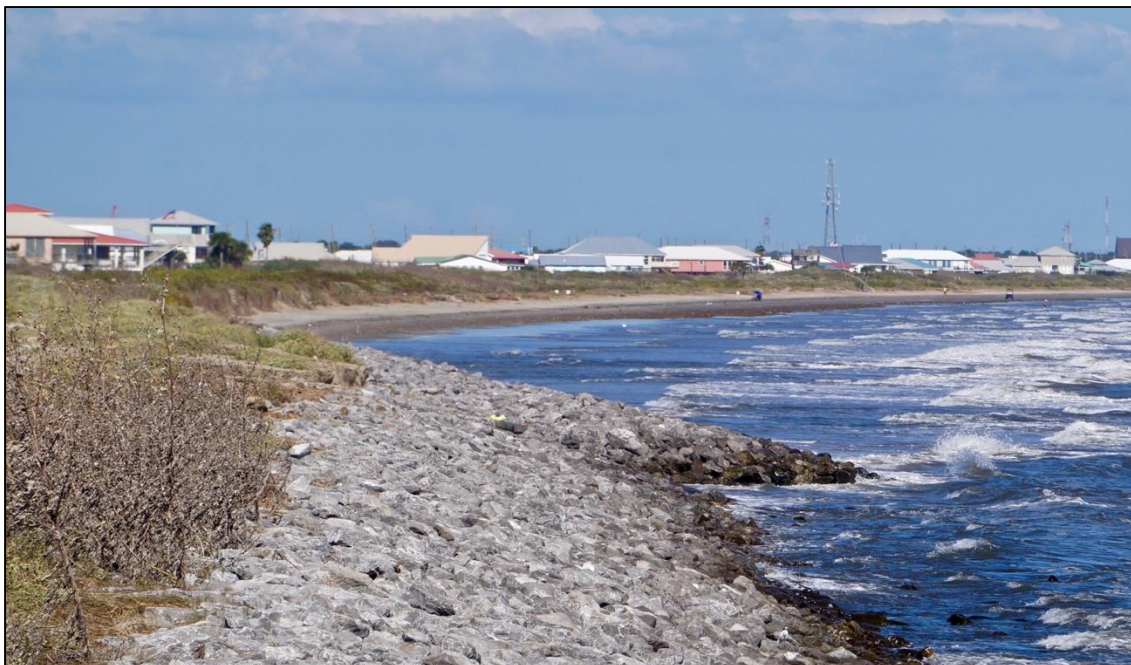
Image 5: Additional rip rap on the western end of the hurricane protection dune with houses built behind the structure. Source: Miller, Lauren 2018.
