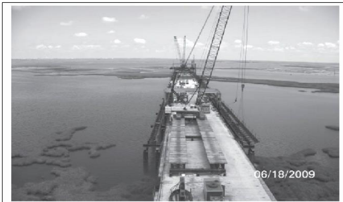
Image 2: Pre-Katrina construction of twenty-two-foot elevated highway LA 1 using the environmentally preferred construction method that eliminates the need for dredging a canal to accommodate heavy-lift cranes. Source: Theriot 2014.
