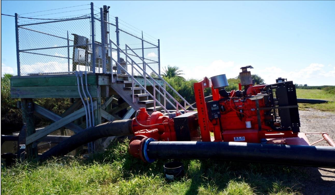
Image 9: Electric drainage pump (left) and diesel pump (right) at the bayside of Grand Isle, Louisiana. Each pump works to pump floodwaters away from the community and over the tidal surge protection levee during storms and other events. Source: Miller, Lauren 2018.
