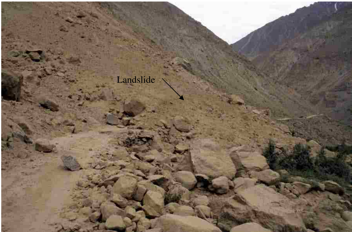
Figure 36. A landslide blocked the road between Askole and Chakpo in the Braldu Valley after heavy rainfall in July 2005.
