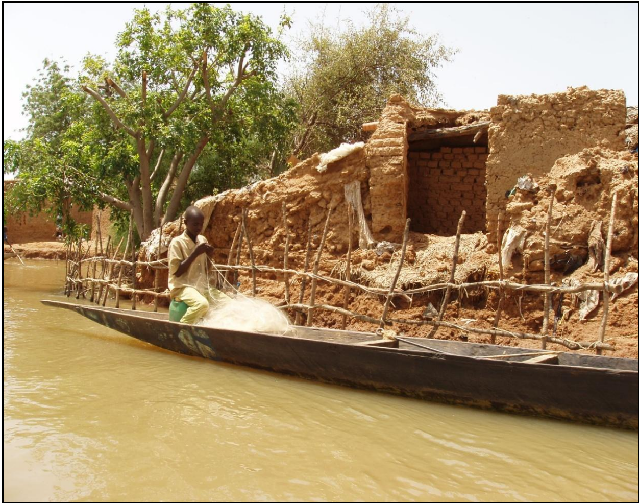
Figure 8. During the rainy season village banks are eroded away by the high water levels. This photo was taken from the Niger River looking at the eroding banks of Dangueri Maliki. Erosion barriers are put into place (wood fence as seen in photo). However, these efforts appear to do little in the way of stopping village erosion (Source: Ashley Williams, 2009).
