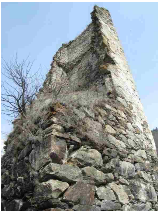
Figure 16. The fragments of the last Svan tower in Mazeri (Photo by Peter Bordokoff, April 2013).
