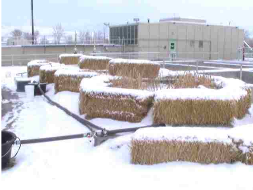
Figure 30. Photo of the experimental system during the winter. Exposed plumbing was wrapped with a heating wire and insulation. This prevented the freezing of pipes and valves under the wintertime operating conditions.
