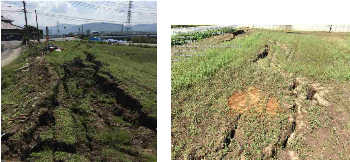
Figure 6-26. Hypothesized lateral spread at site 4 and observed fissures and ejecta (Kayen et al., 2017)
