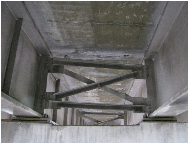
Figure 4-20: Insignificant efflorescence and cracking on the underside of the deck in case study #2.
