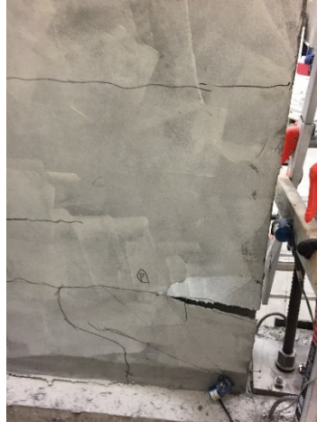
(b) Toe crushing.
