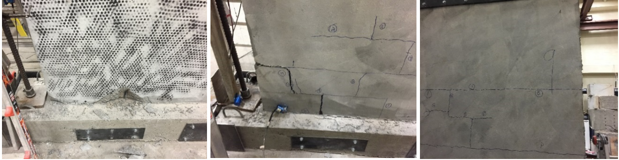
(a) Failure at connection. (b) Diagonal cracking. (c) Lack of cracking in top of wall.
