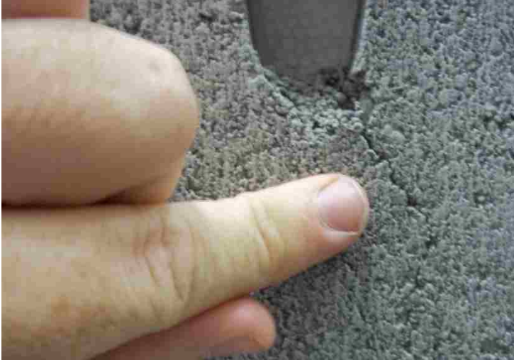
Figure 4-7 Cracking in web prior to testing.
