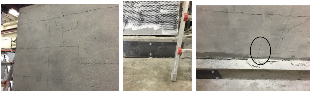
(a) Typical cracking.
