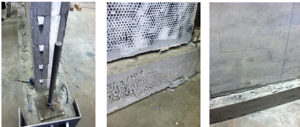
(a) Cracking of outside webs. (b) Uplift of wall. (c) Diagonal cracks.
