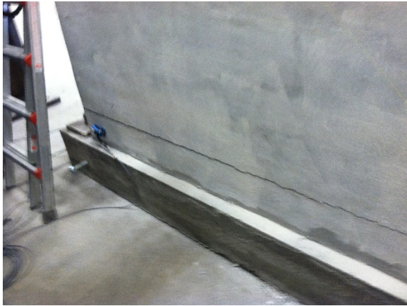
(a) Horizontal crack close to actuator.
