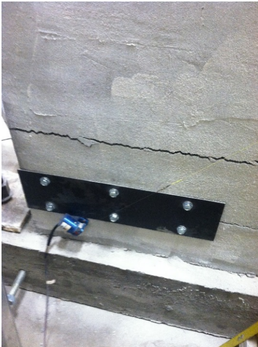
(a) Horizontal crack above steel plate.
