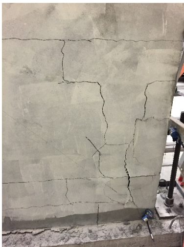
(a) Toe crushing.
