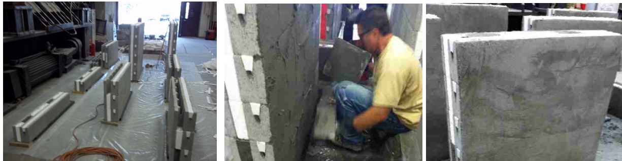
(a) Stacking the wallettes. (b) application of structural coat (c) Finished wallettes
