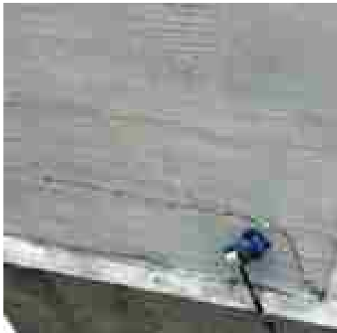
(a) Toe crushing and horizontal crack.
