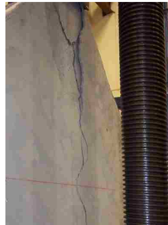
(c) Crack on face.
