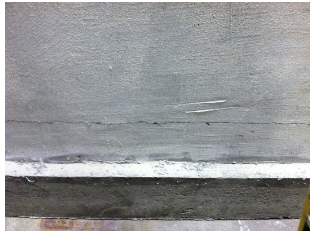
(b) horizontal crack.
