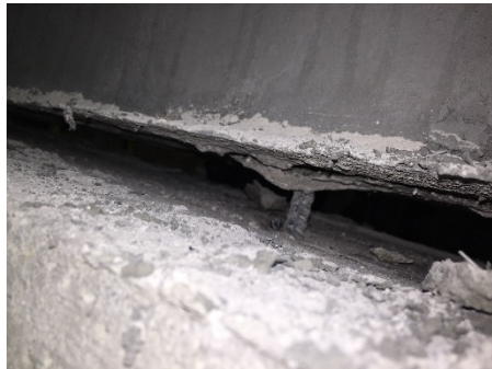
(a) Wall uplift.
