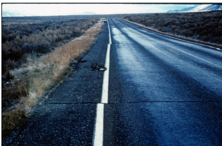
Figure 6-3. Photograph showing lateral displacement of Highway 93 near the 1985 Whiskey Springs investigation site (Youd et al. 1985).
