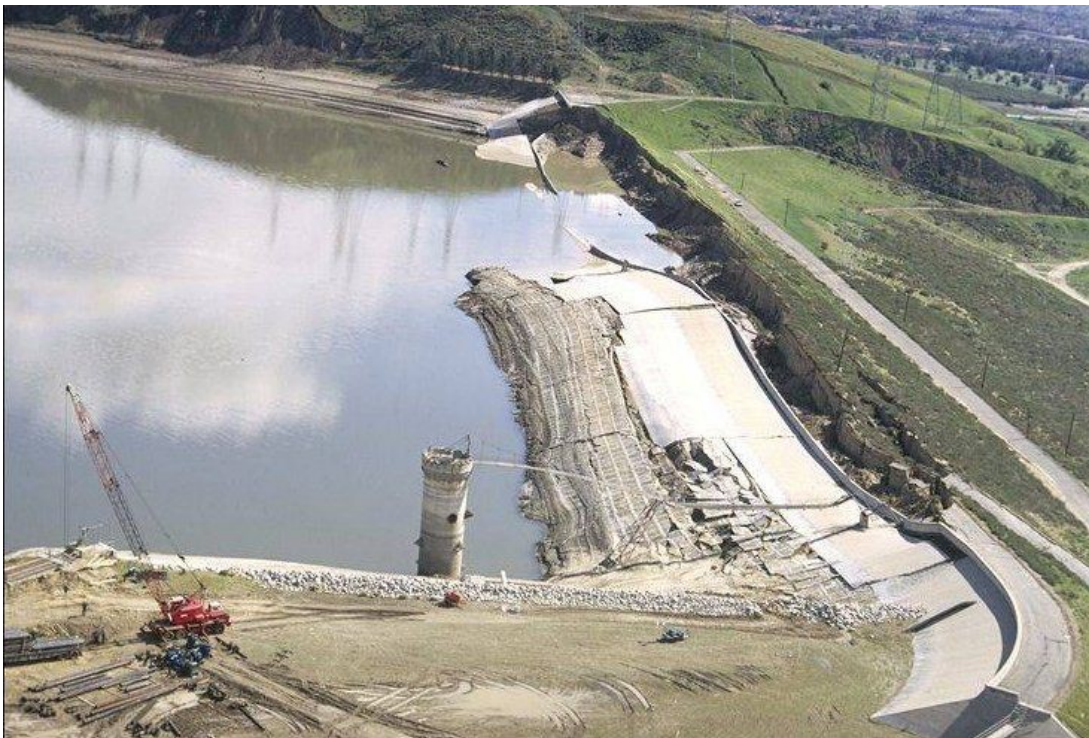
Figure 3-15: Flow liquefaction failure of the Lower San Fernando Dam, 1971 (courtesy of the National Information Service for Earthquake Engineering, EERC, University of California, Berkeley).
