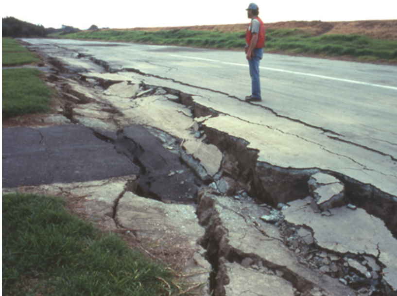
Figure 3-20: Lateral spreading from the 1989 Loma Prieta earthquake.
