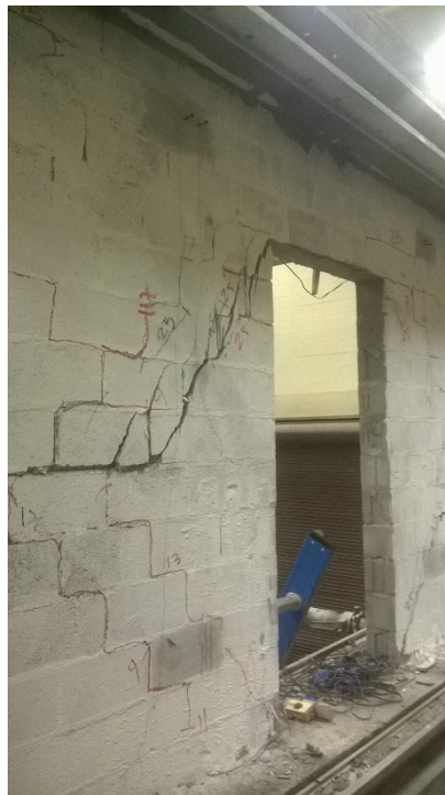
Figure 3-12: Marking Cracks During Testing
