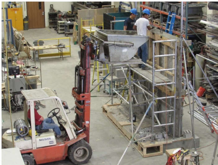
Figure 3-5: Construction of the Walls and Pouring of the Second Story Slab Showing the Scaffolding and Tripods
