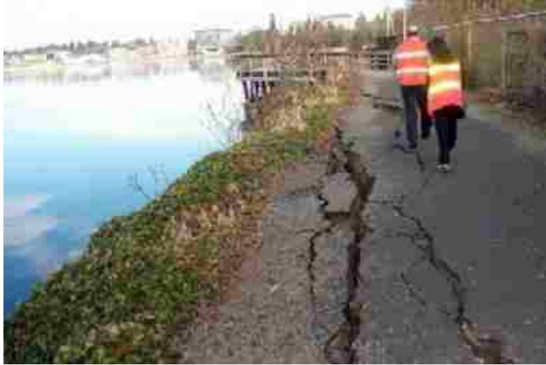
Figure 3-20: Example of lateral spread displacements causing cracking of pavement after an earthquake that occurred in Olympia, WA, in 2001 (after Bray et al. (2001)).
