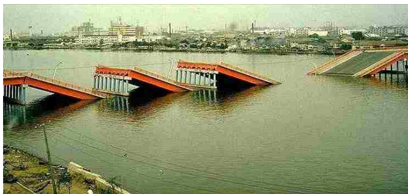
Figure 4-1: Example of lateral spread displacements causing bridge spans of the Showa Bridge in Niigata, Japan, to lose support and collapse in after the 1964 earthquake (after Bhattacharya et al. (2014)).
