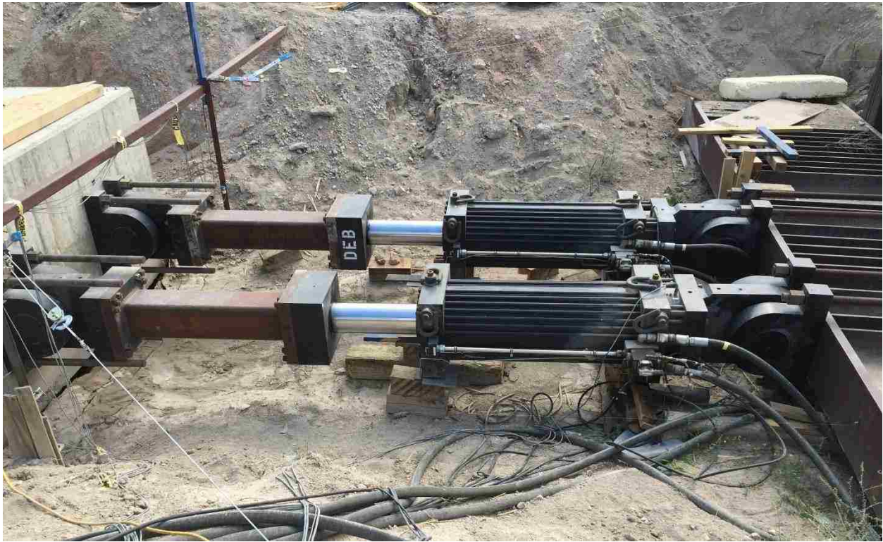
Figure 3-4: Hydraulic actuator setup as viewed from the west side
