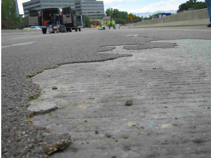
Figure 2-9: Delamination of polymer overlay.
