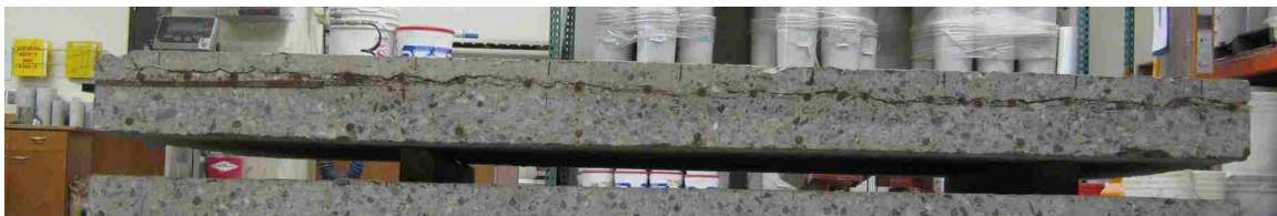
Figure 2-3: Delaminated concrete bridge deck slab.
