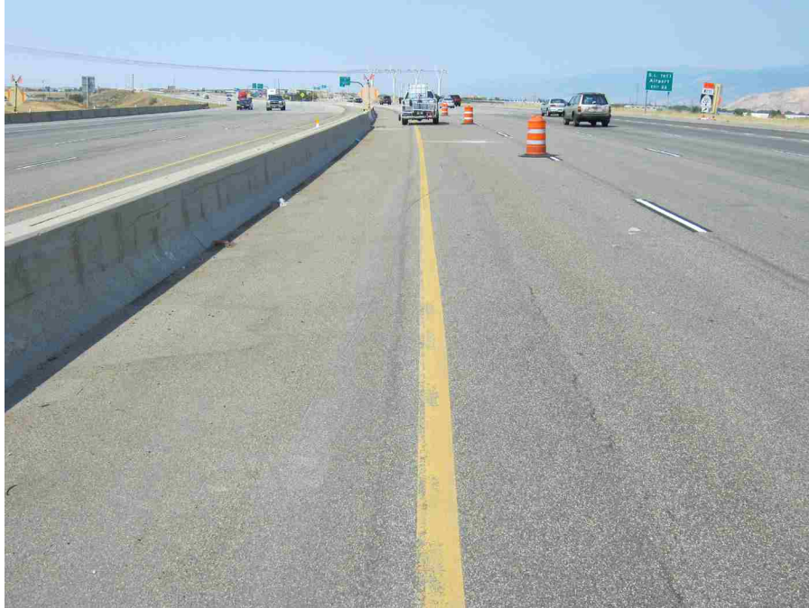
Figure 2-8: Cracking of asphalt overlay.
