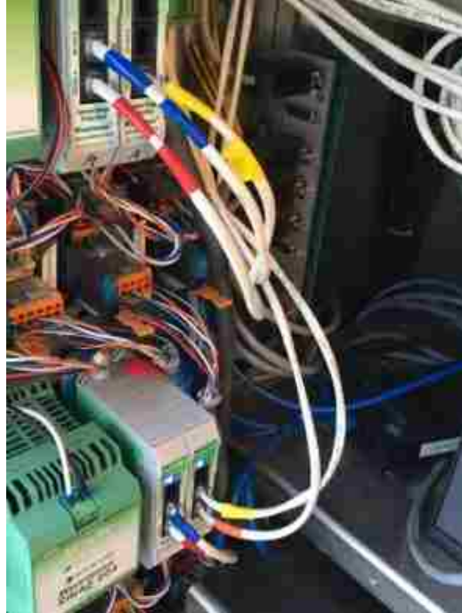
Figure 3-20: Double taped Advance cables with bridge ports above the cables (photo taken by Greg Sanchez).
