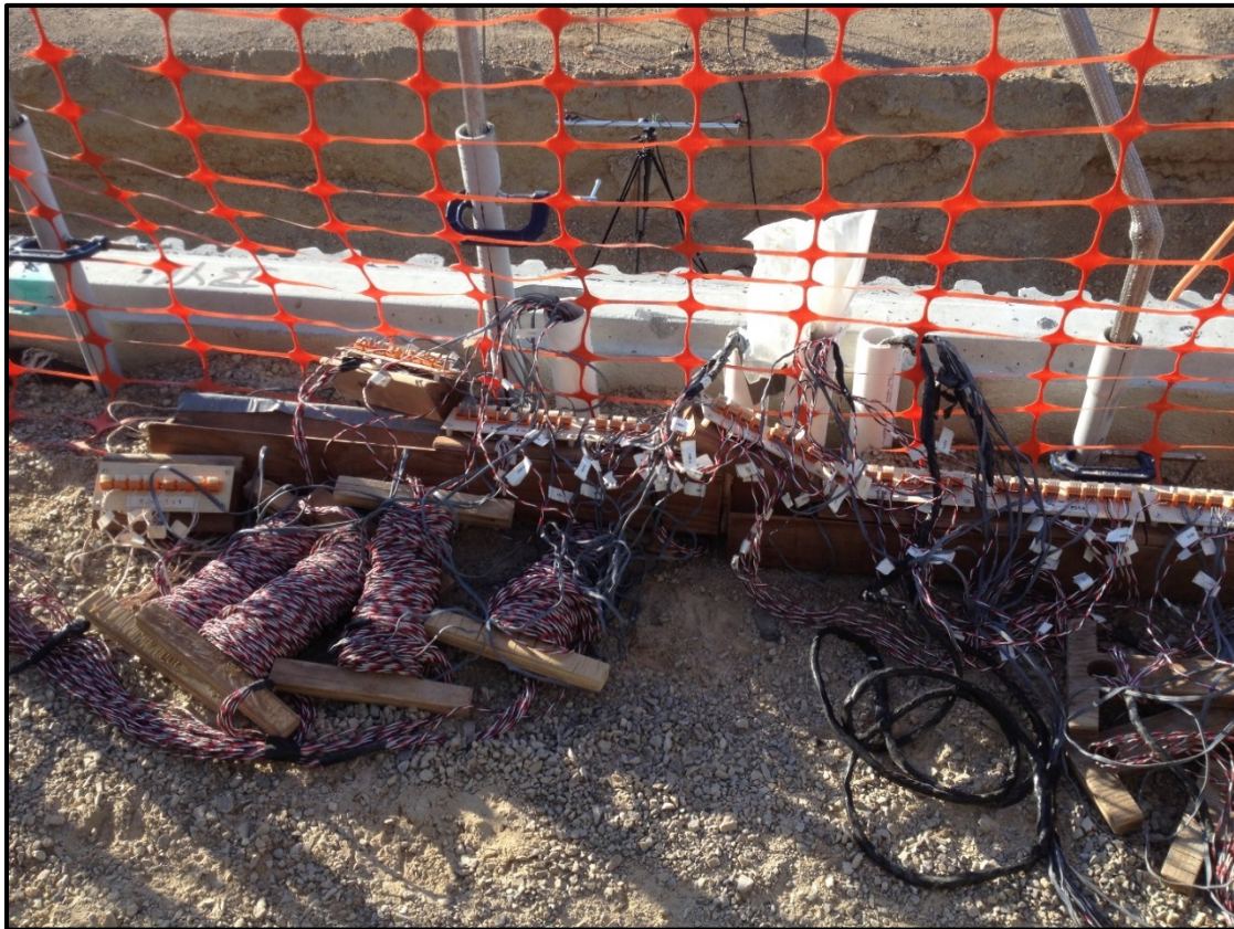
Figure 4-4: Strain gauge connections to terminal strips.
