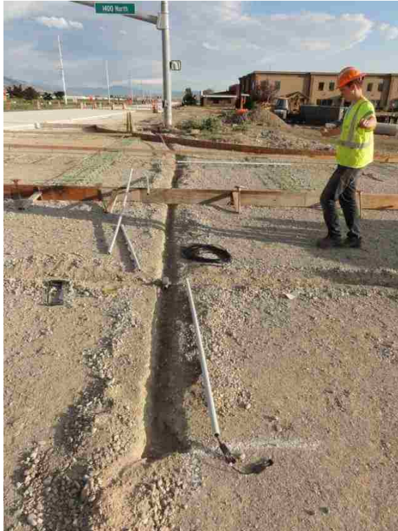
Figure 3-5: Sensor cables in PVC pipe.
