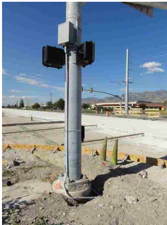
Figure 3-6: Utility box mounted on signal pole.
