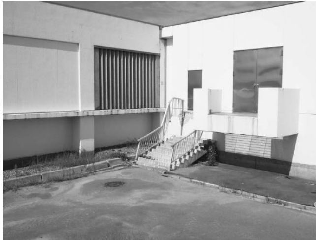
Figure 5-3: Collapsed stairway resulting from settlement (after Tsukamoto and Ishihara 2010)
