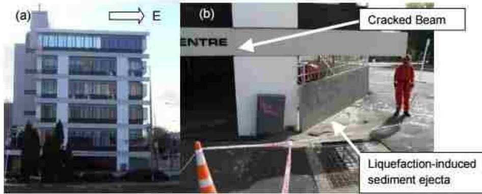
Figure 5-4: (a) Building tilt and (b) structural damage resulting from differential settlement (after Bray et al. 2013)
