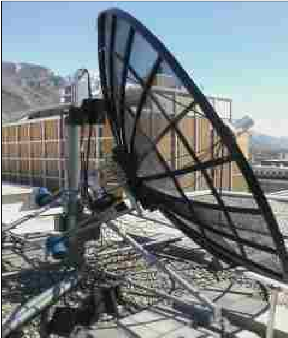
Figure 3-8: Antenna broken and blown off its azimuth/elevation mount as a result of a gale-force windstorm. Photo is courtesy of the author
