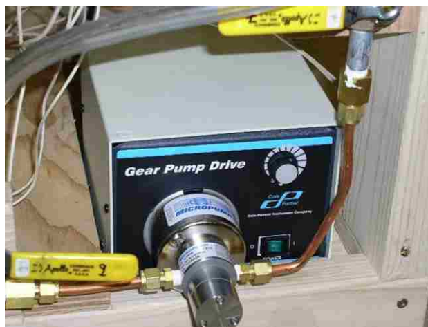
Figure 21. Liquid Pump, P-101.
