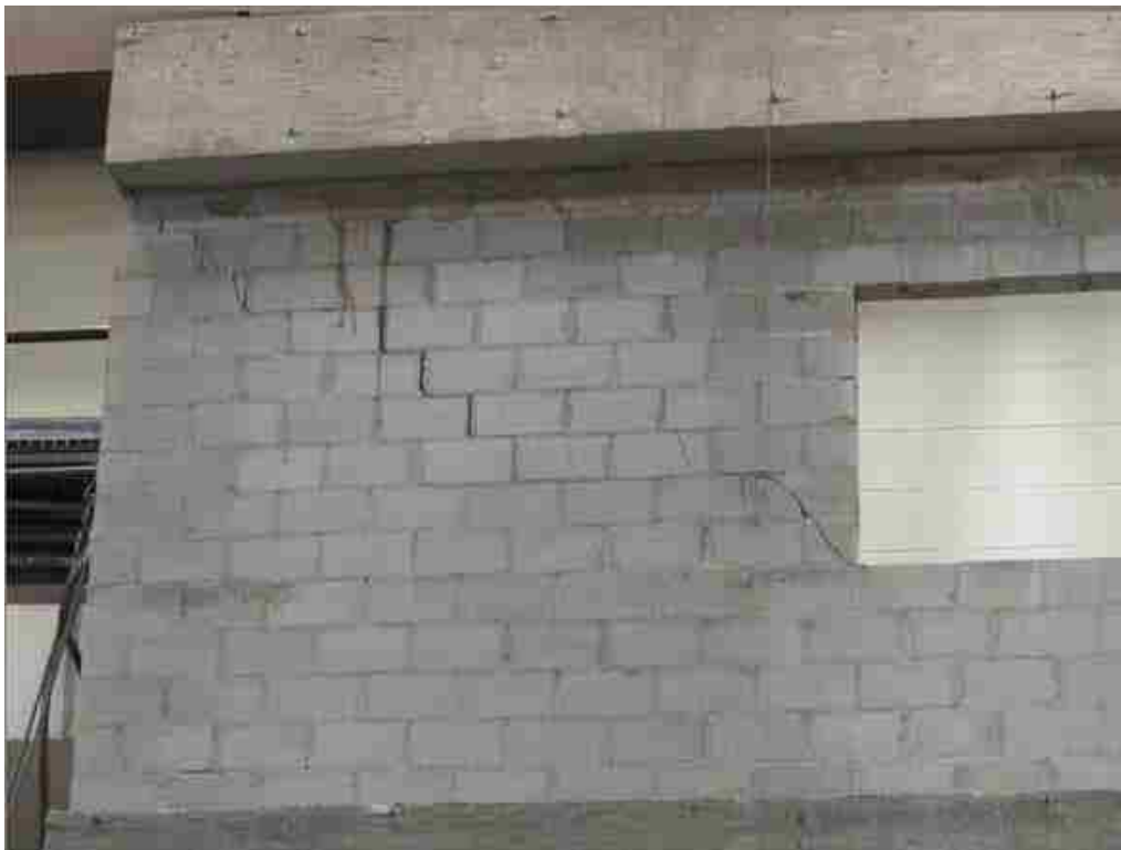
Figure 4-6: Diagonal cracks stepping through mortar joints
