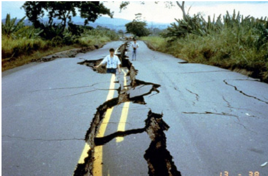
Figure 3-17: Liquefaction and Lateral Spreading Induced Fissures in the Main East-West Highway between Siquerres and Puerto Limon (ERI, 2016).
