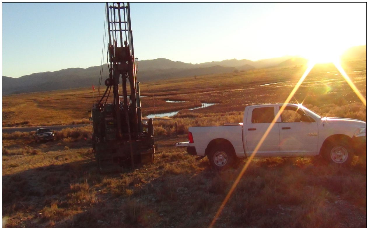
Figure 6-7. Photograph showing site conditions at Whiskey Springs in 2015 near BC3, looking southwest. Highway 93 can be seen in the background.
