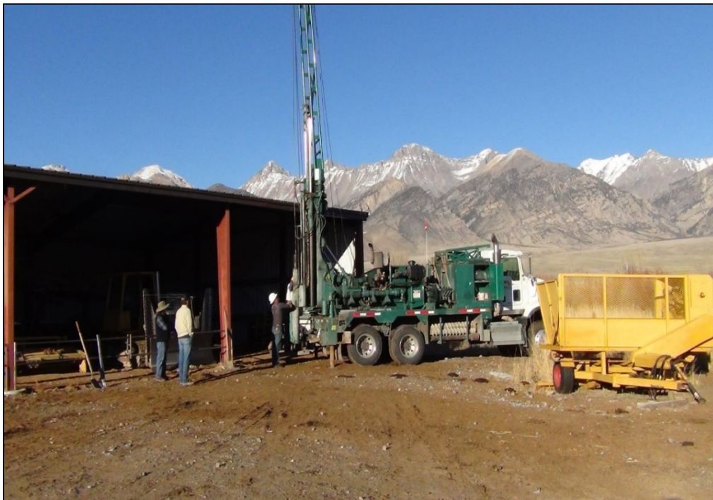
Figure 5-6. View looking northeast showing CME rig set up at Pence Ranch site near BPC-B, November, 2016. Shed is of recent construction.
