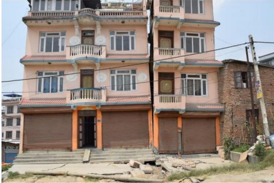
Figure 3-12: Damage to a Building due to liquefaction-induced differential settlement in Kathmandu, Nepal from 2015 earthquake event (after GEER, 2015).
