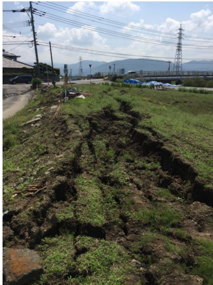
Figure 3-13: Lateral Spread visible near Kathmandu, Nepal after 2015 earthquake events (after GEER, 2015).
