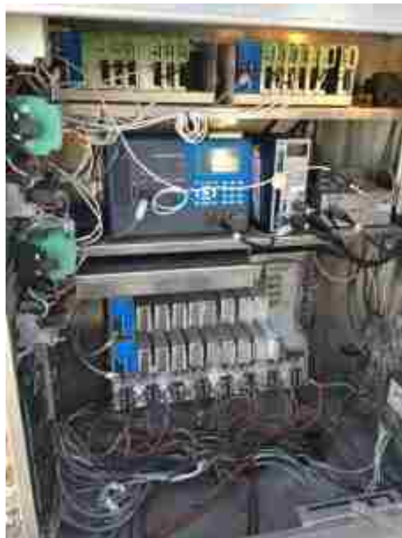
Figure 3-19: Image of the inside of a traffic controller box (photo taken by Greg Sanchez).
