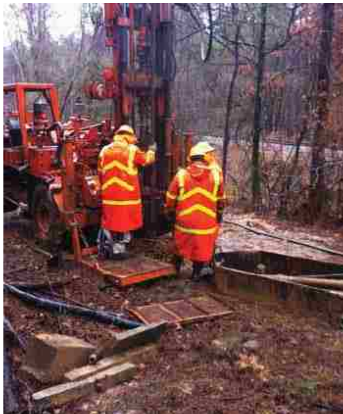
Figure 3.1-3 Photo of the drill rig for the standard penetration test (SPT) (Bey 2014).
